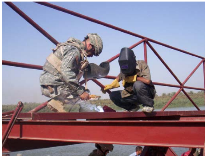
Sgt. Russell Dinkins of Darien works with Iraqis on a major construction project.
